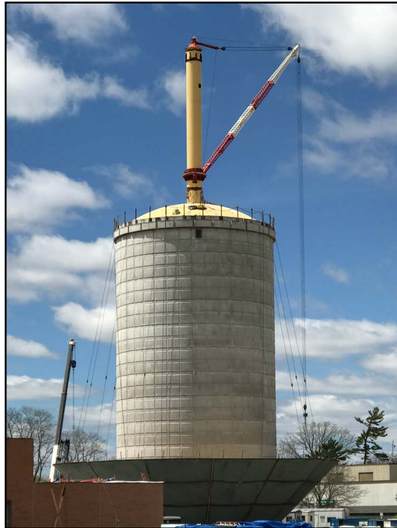
The new water tower and treatment facility are being built near the power plant on Service Road with an early 2020 completion date.
