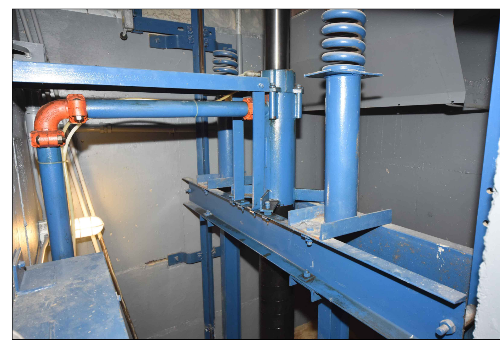
3 A5.2 ELVTR. EP2 STEEL FRAMING FOR ELEVATED JACK AND BUMPERS AT PIT NO SCALE
