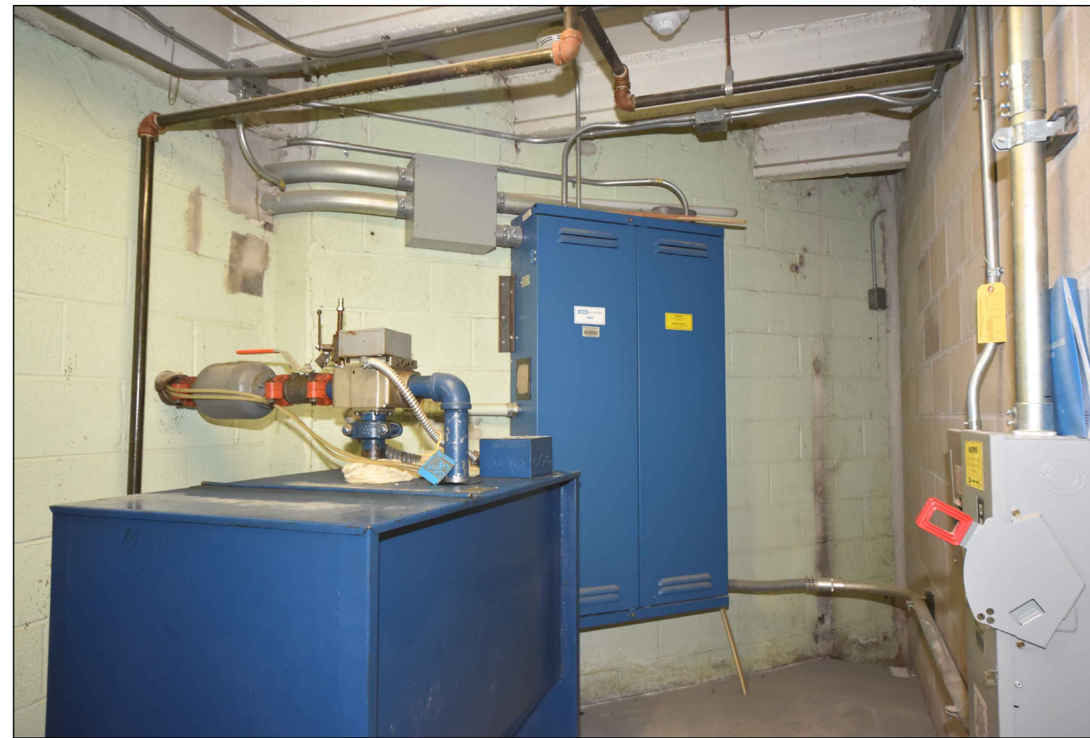
2 A5.1 EXISTING MACHINE ROOM AT ELEVATOR EPI NO SCALE
