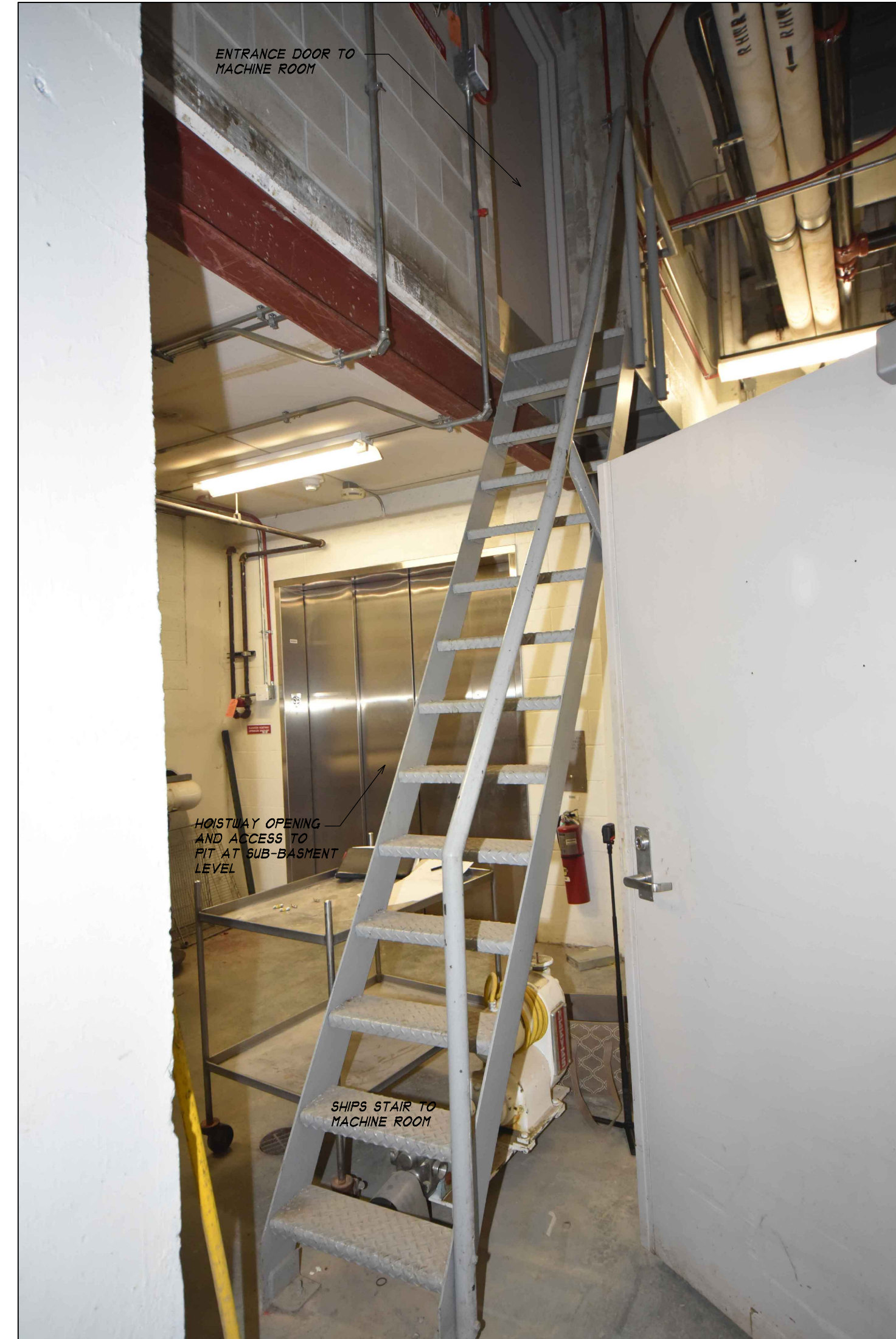
5 A5.3 SUB-BASEMENT LEVEL ACCESS TO MACHINE RM. AND PIT - LEVATOR EP3 NO SCALE
