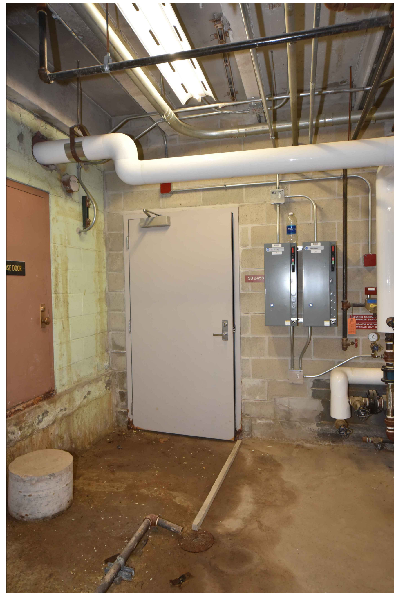
4 A5.1 EXISTING ENTRANCE TO MACHINE ROOM AND PIT AT SUB-BSMT. - ELEVATOR EPI NO SCALE
