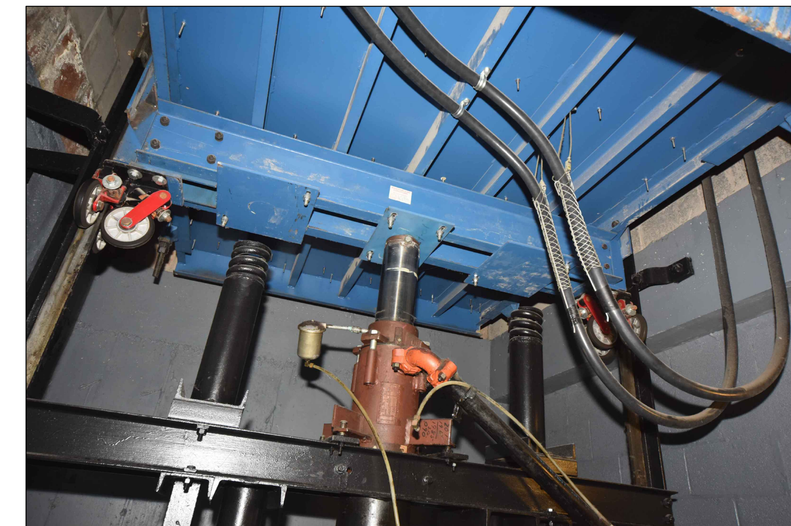
3 A5.1 ELVTR. EPI STEEL FRAMING FOR ELEVATED JACK AND BUMPERS WITH SLING AND FLOOR FRAMING NO SCALE
