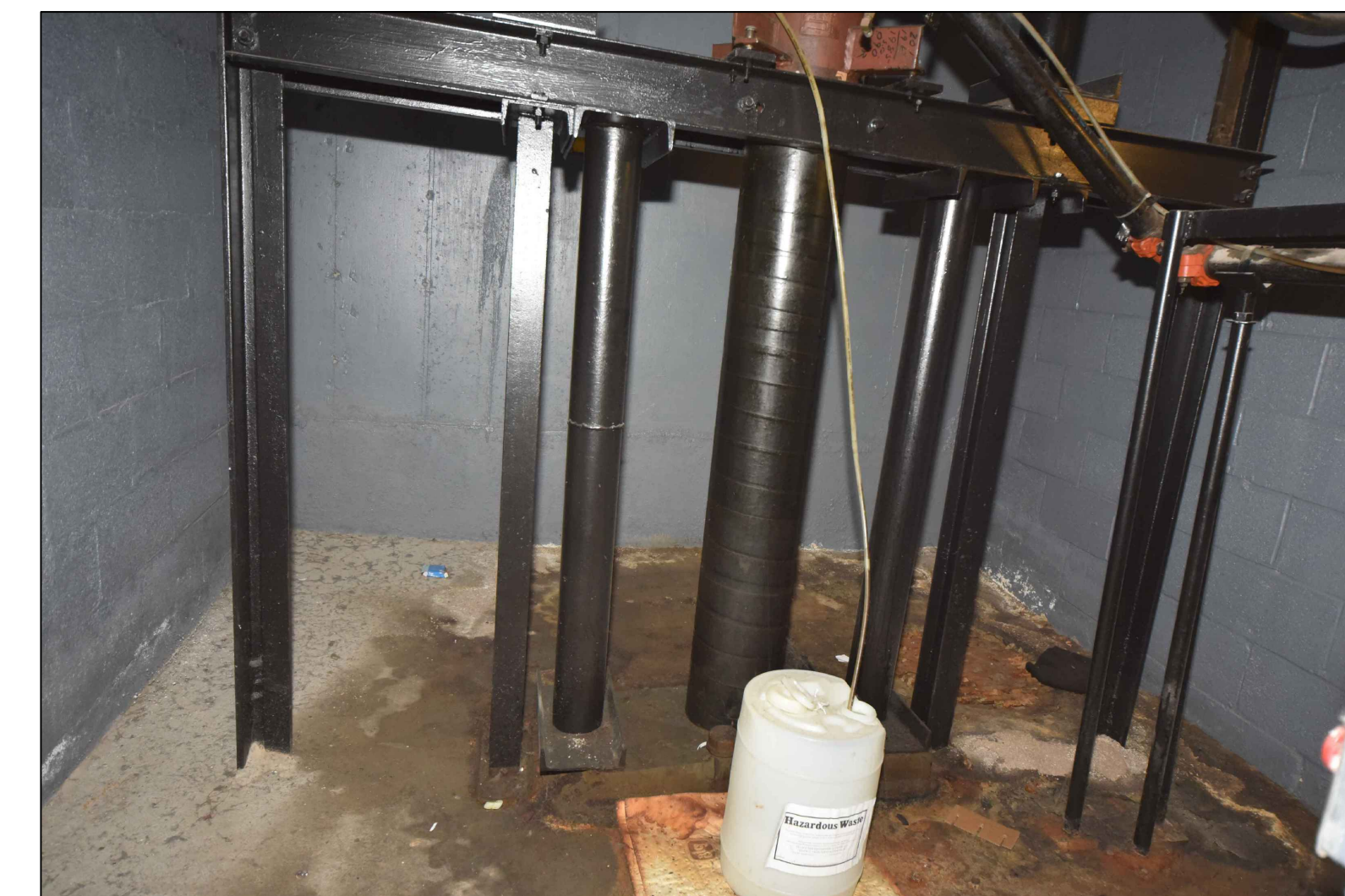
4 A5.1 EXISTING STEEL FRAMING FOR ELEVATED JACK AND BUMPERS AT PIT FLOOR - ELEVATOR EPI NO SCALE
