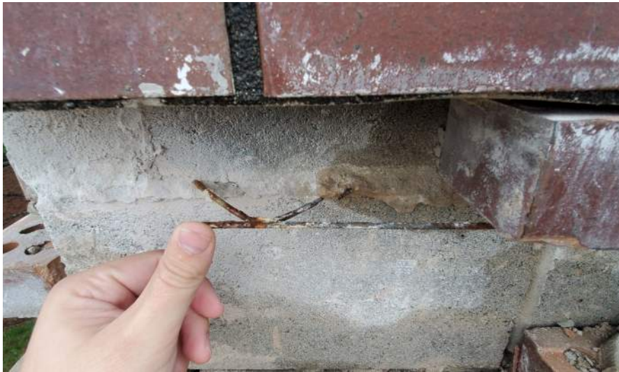
Brick ties are corroded and broken from back wall.
