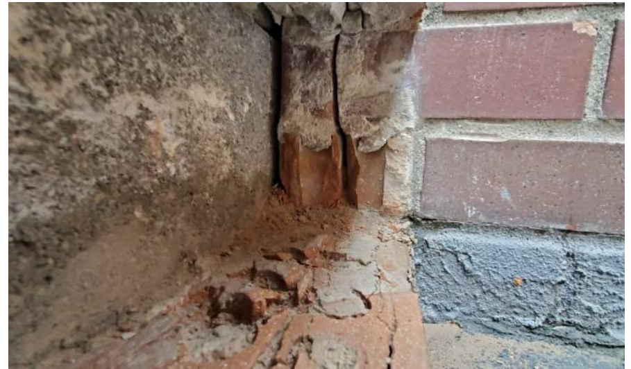
Brick in the parapet wall is cracked through the middle.
