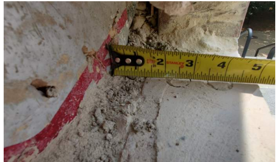
One and a quarter inch gap between building insulation and brick veneer.
