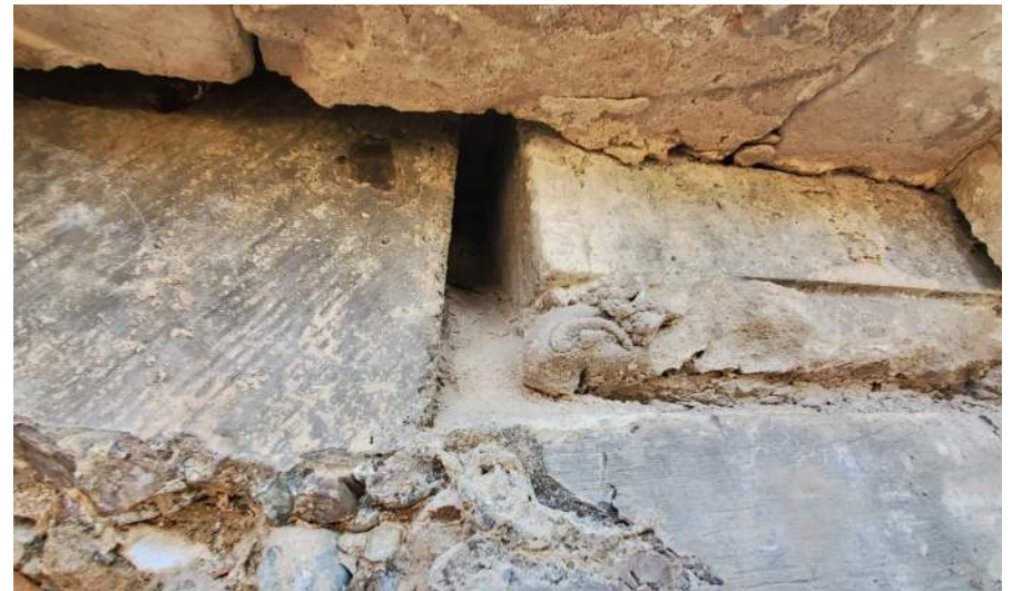
Large open void between CMU back wall and concrete stair.
