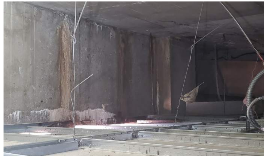
Water staining where the plaza intersects with the building.
