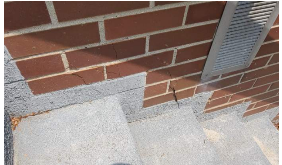
Small areas of damaged brick where the stairs meet Wharton Center.
