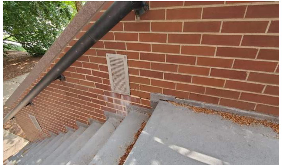
Deteriorated brick and mortar around lights.
