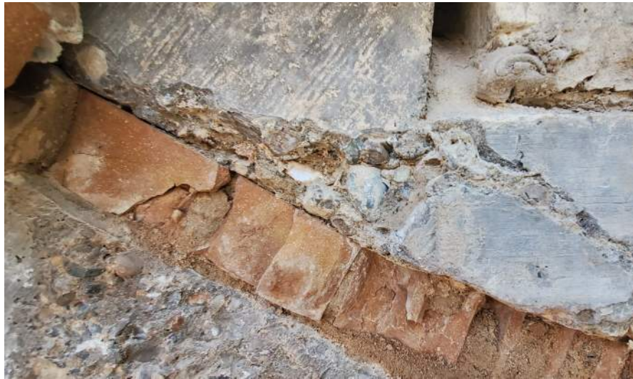
Brick and sand used as a cold joint between Plenum ceiling and stair.
