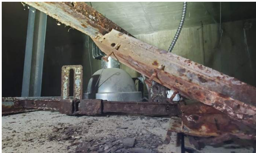
Soffit structure and light corroded from drain water.
