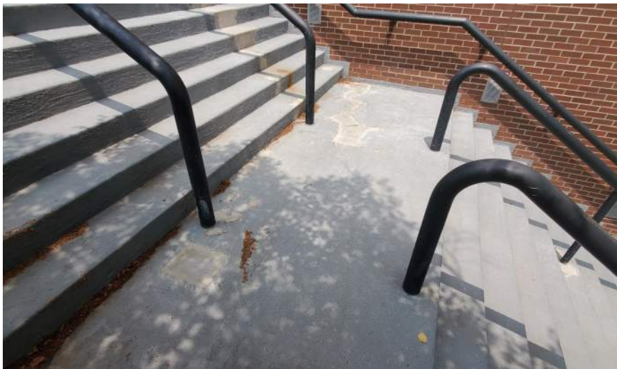
Cracked coating in the stair landing and repairs to the stairs.
