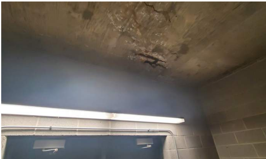
Damaged ceiling in the utility stairway under the Plaza.
