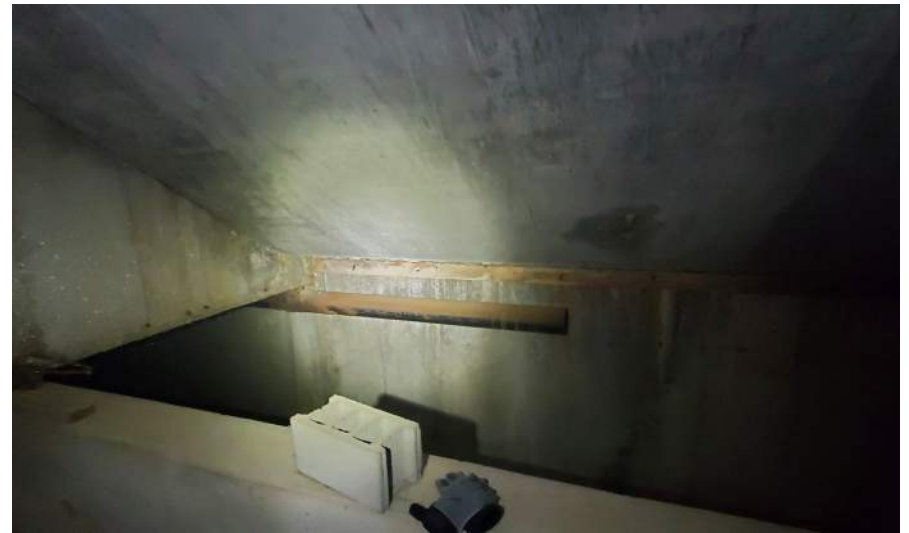
Water staining along the back plenum wall under stair landing,
