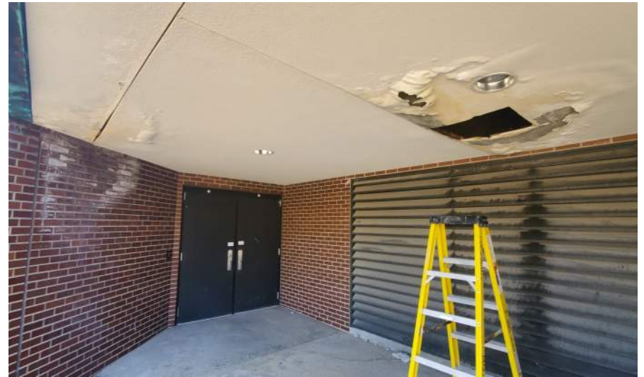
Damaged soffit under Plaza.
