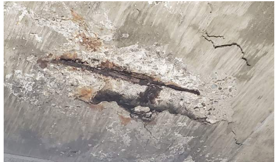
Corroded reinforcement in the utility stairway ceiling.
