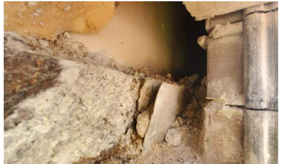
No flashing installed over lintel vertical leg.
