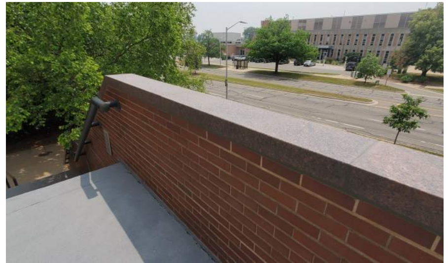
Granite coping cap is in good shape and can be reused.
