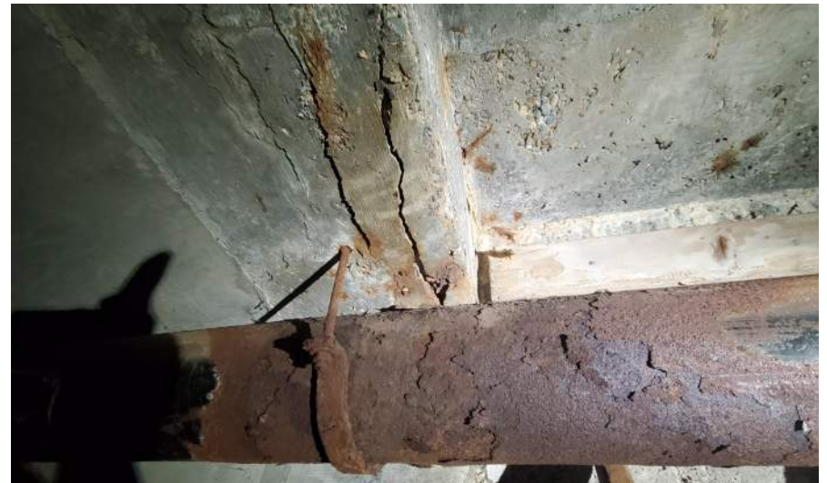
Damaged ceiling Intersection of plenum where stairs meet the building,
