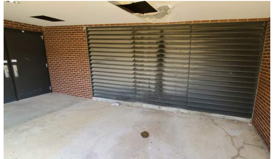
Drain leaking through soffit opening.
