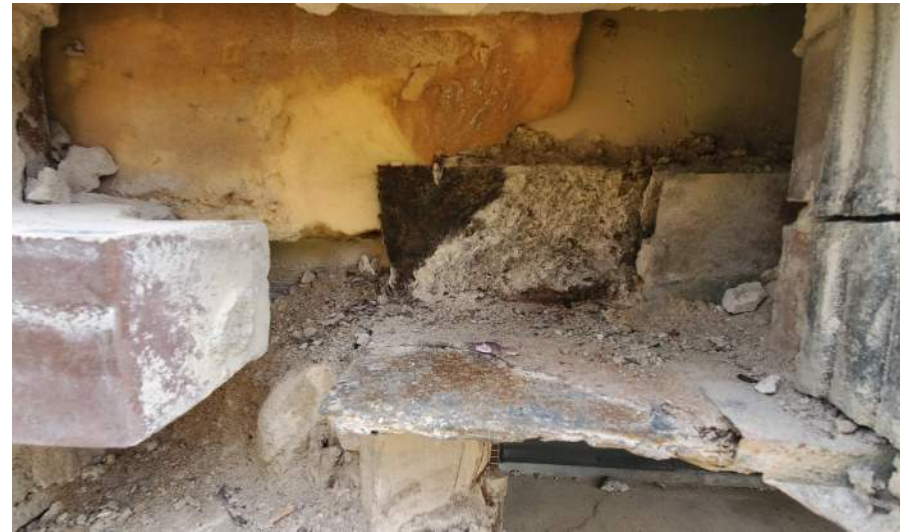
Lintel end vertical leg is heavily corroded.
