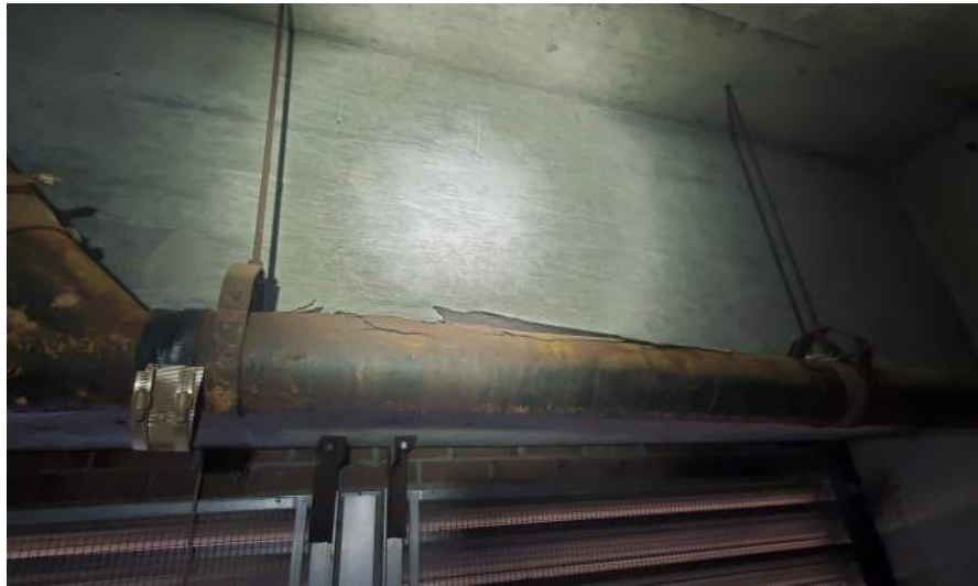
Corroded Plaza drain pipe in the plenum.
