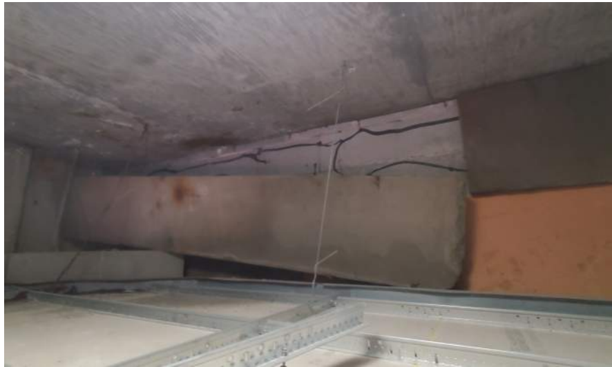
Building insulation has fallen in the soffit space.
