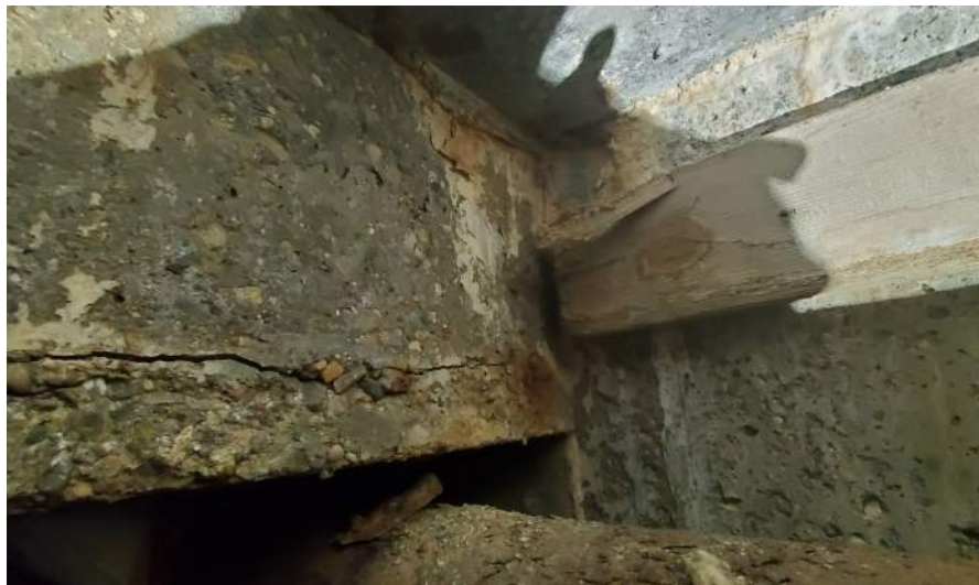
Damaged ceiling intersection of plenum where stairs meet the building.
