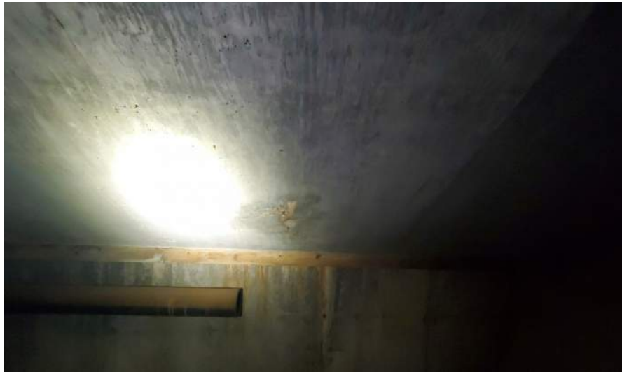
Small spot of reinforcement corrosion in the plenum ceiling.
