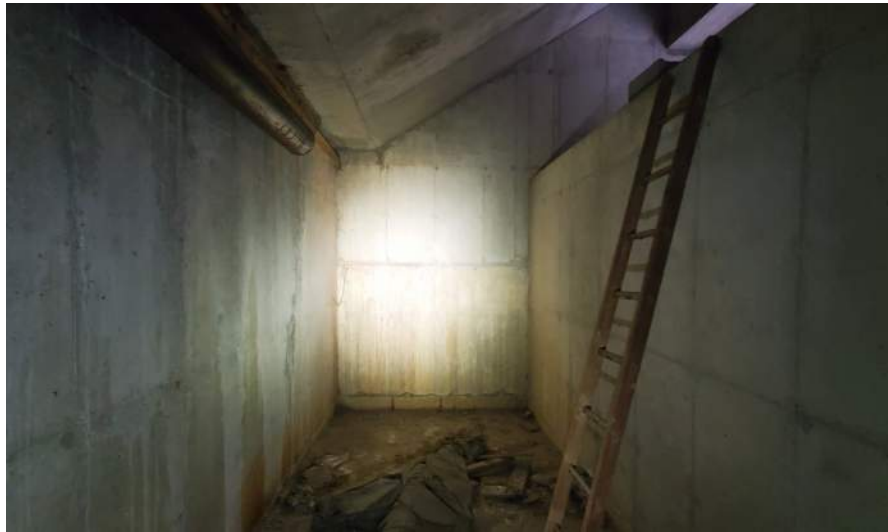
Plenum under the stairway overview.
