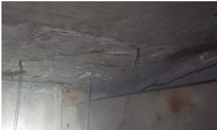
Corrosion in the ceiling structure above soffit space.
