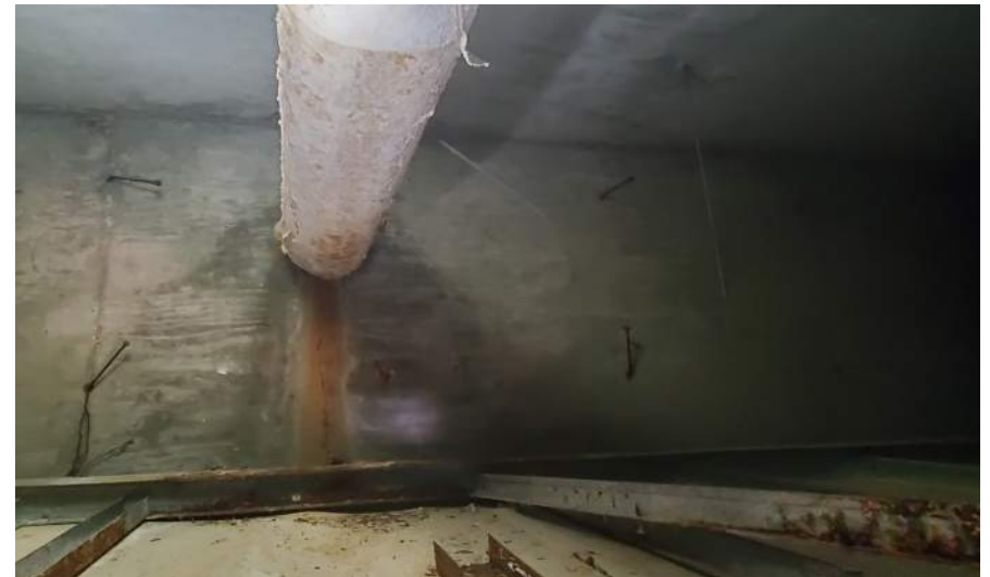
Plaza drain pipe is insulated in the soffit space, but not the plenum space.
