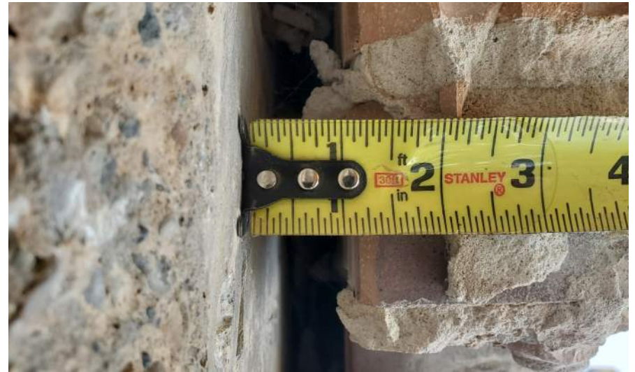
One inch gap between brick veneer and cast-in-place concrete back wall.
