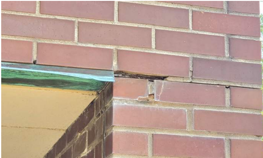
Lintel end opposite the masonry opening is corroded and damaging area.
