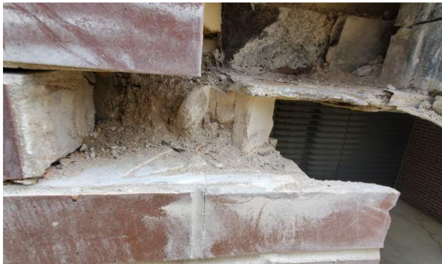
Lintel is about six inches short of sitting on structural CMU back wall.
