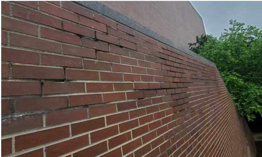
Deteriorated mortar at the top of the stair exterior wall.
