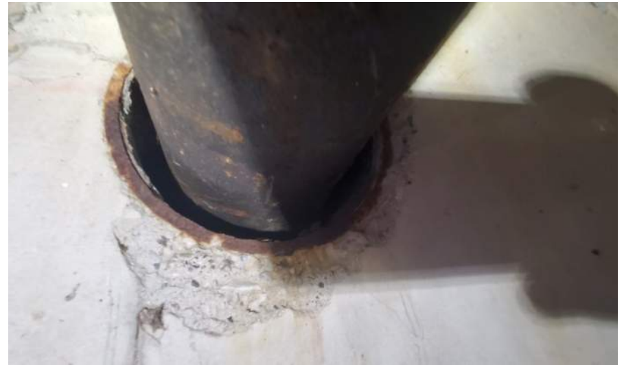
Plaza drain pipe drains into Wharton Center through plenum.
