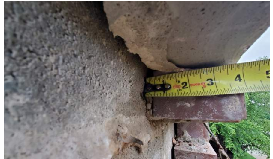
Less than a half inch gap between brick veneer and CMU back wall.
