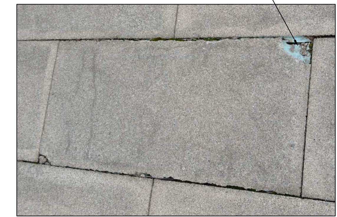
REINSTALL PANEL PANEL CAN BE RE-INSTALLED FOLLOWING PATCH AND REPAIR; REFER TO TECH NOTE IN PROJECT MANUAL
