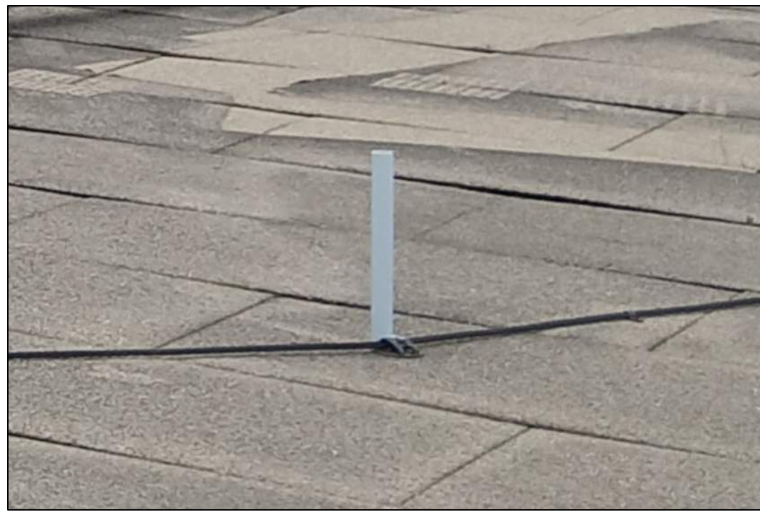
DECK MOUNTED LIGHTNING PROTECTION
