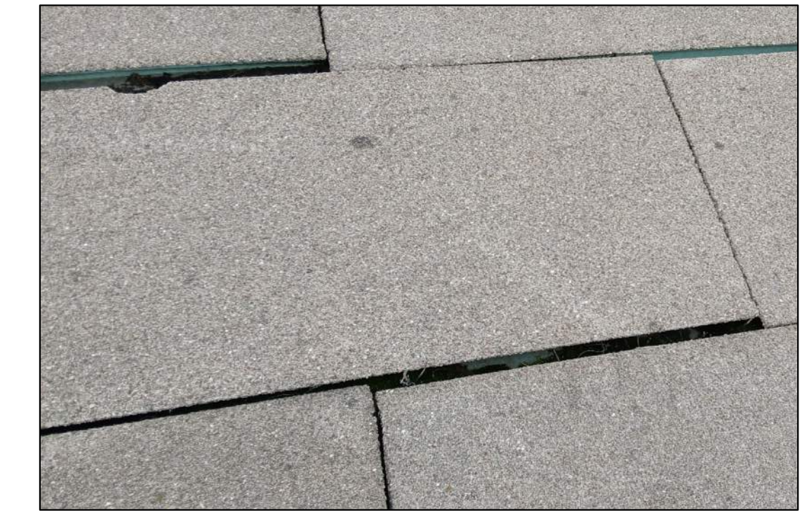
REINSTALL PANEL PANEL CAN BE RE-INSTALLED FOLLOWING PATCH AND REPAIR; REFER TO TECH NOTE IN PROJECT MANUAL
